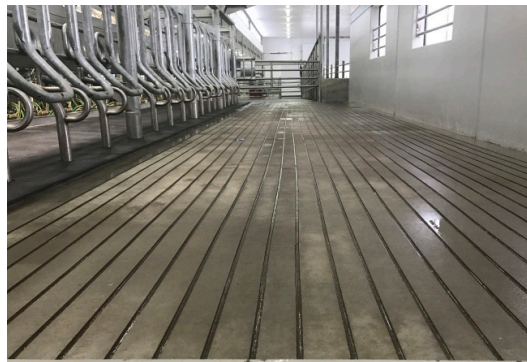
Texturing was done by rake across the plastic concrete surface for a friction finish for animal traction and welfare.
