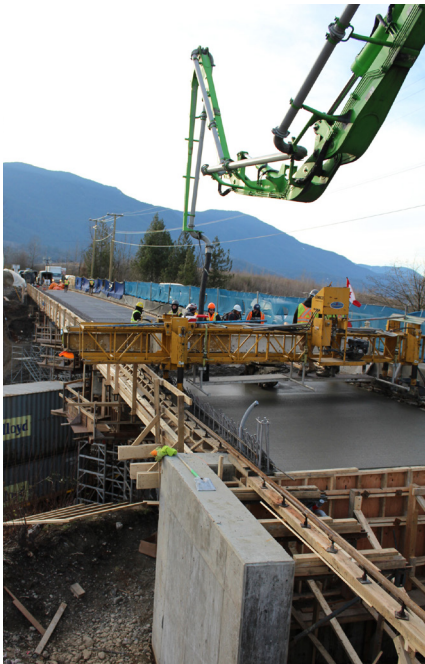
Krystol Internal Membrane™ (KIM®) was added to the concrete mix for this bridge deck to permanently waterproof it.
