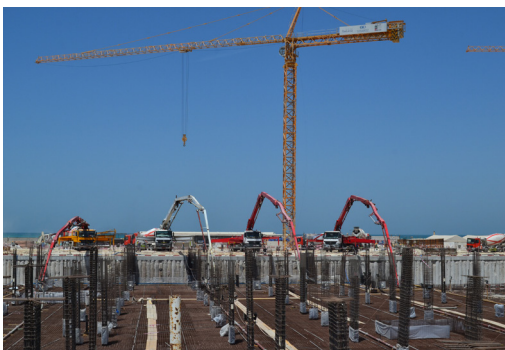
More than 18,700 m 3 of KIM concrete was poured in the foundation of the hotel.
