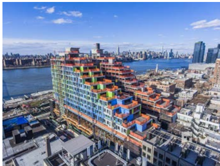
The first of five waterfront buildings waterproofed with KIM Admixture in the shotcrete walls.
