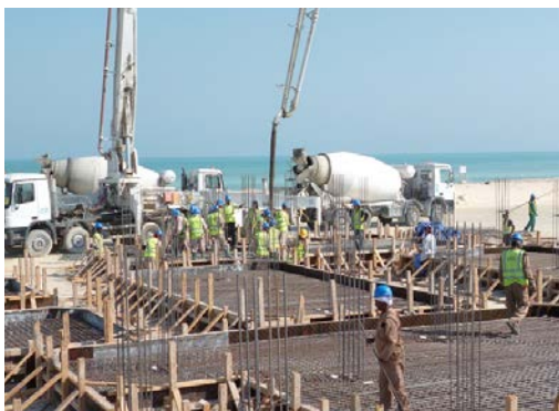
KIM concrete was used to waterproof the isolated footings, grade beam, column neck, and water retaining structures.
