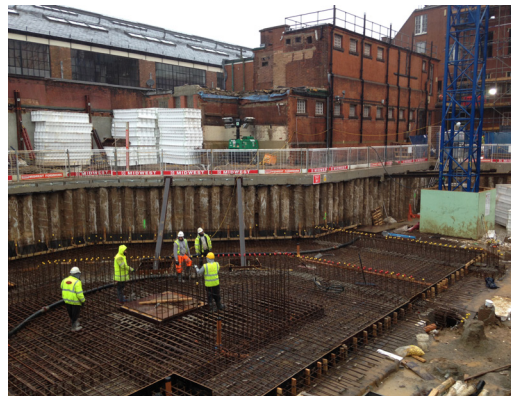
Using Kryton's Krystol Waterstop system, the project was protected from corrosion of rebar.
