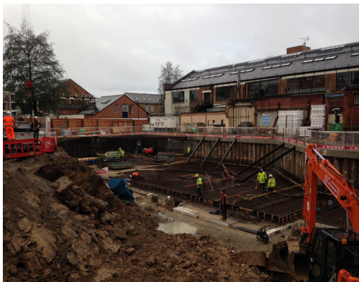
Over 1000 m 3 of KIM treated concrete was used for the basement slab and walls.
