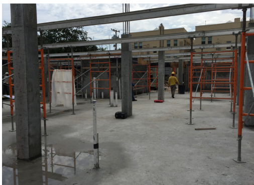
KIM concrete was used in the foundation slab, all columns, and the elevator pit.
