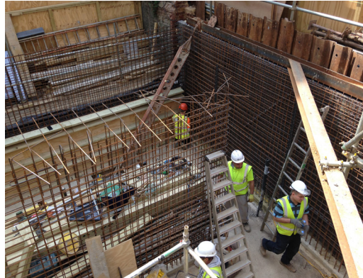
Krytonite Swelling Waterstop was installed between the rebar to ensure a fully tanked basement.
