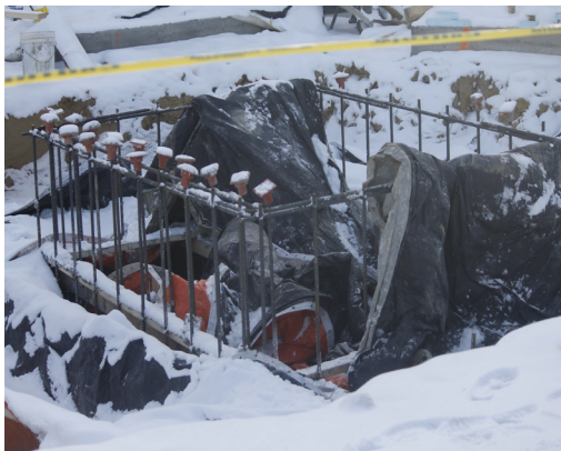
KIM was originally to be used just for the elevator pits, but was extended to the foundation as well.
