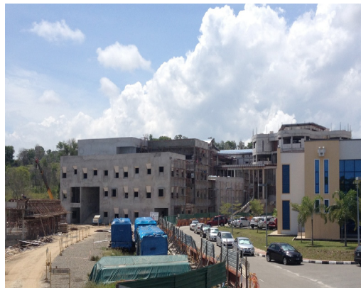
Over 2, 850 m 2 (30, 677 sq/ft 2 ) of Krystol T1 & T2 was used to waterproof the concrete.
