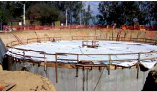
TreePeople Center Underground Cistern, Los Angeles, California, USA
