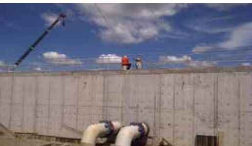
Batu Kitang Water Treatment Facility Complex, Batu Kitang , Kuching, Malaysia
