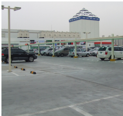
The exposed rooftop slabs relies on KIM admixture for complete waterproofing protection.
