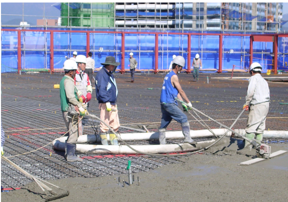
Kryton's KIM was used to improve the workability of the concrete in the suspended rooftop slabs at all HomePlus locations.
