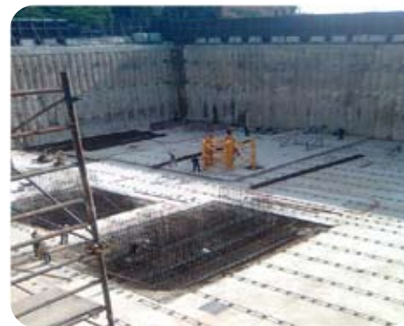
The construction team saved time & labour by using Kryton's Krystol line of products.
