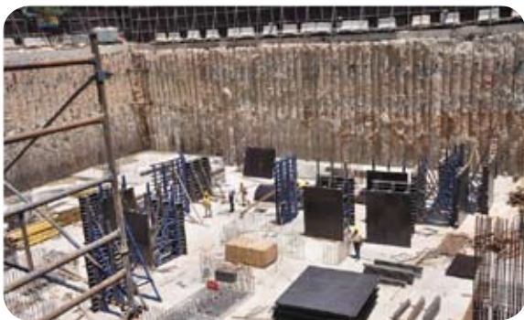
Kryton's products can withstand the high hydrostatic pressure in the area.
