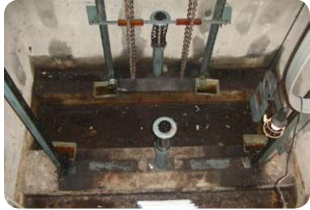
High hydrostatic pressure caused leaks in the elevator lift pit.
