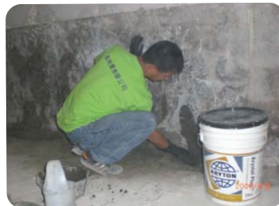
Application of Krystol Plug, as per step #2 of the Crack Repair System
