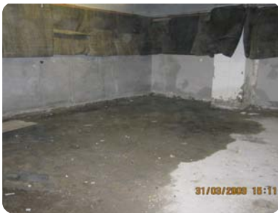
Before: Severe water leakage from the basement walls
