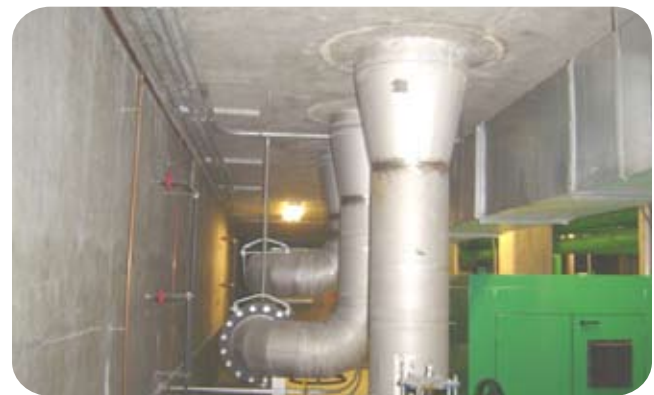
The space immediately below the containment tank houses equipment and must remain completely dry.
