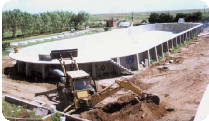
Huge sediment tank is larger than a football field.
