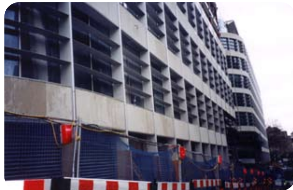
Tower Place is situated near the Thames River, which caused leaking deep in the basement.
