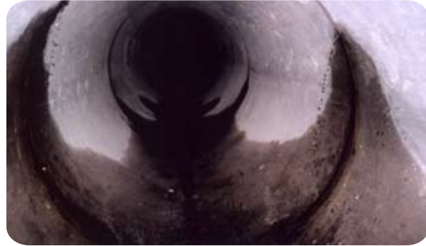
Flowing water on right is visibly active before repair.
