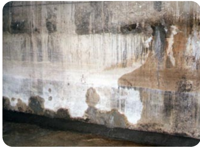
Severe leakage through the walls and joints of the Sewage Pumping Station.
