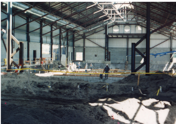
The 57 metre pool has an 18 foot dive tank that is 10 feet below the water table
