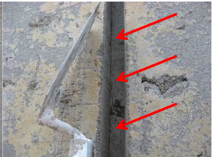
Joint keyway with crack
