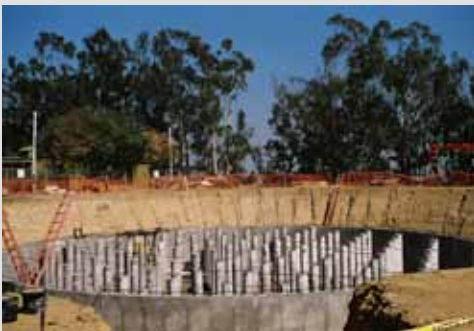
TreePeople Center Cistern, USA
