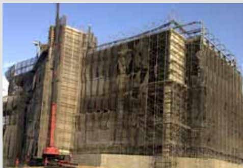
Tong Ho Steel Plant, Taiwan
