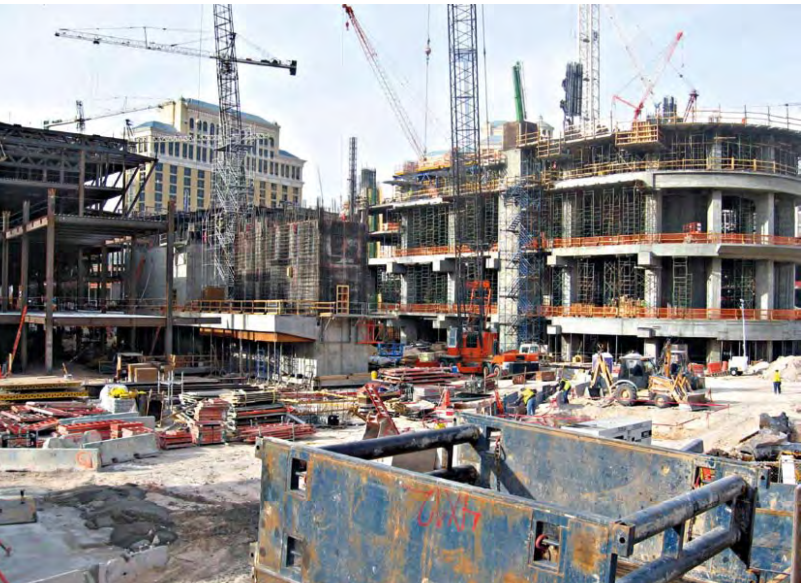
With five buildings going up at different rates, all with a common foundation, and a need to interface these elements with the existing Las Vegas structures, the waterproofing needs were both numerous and challenging.
