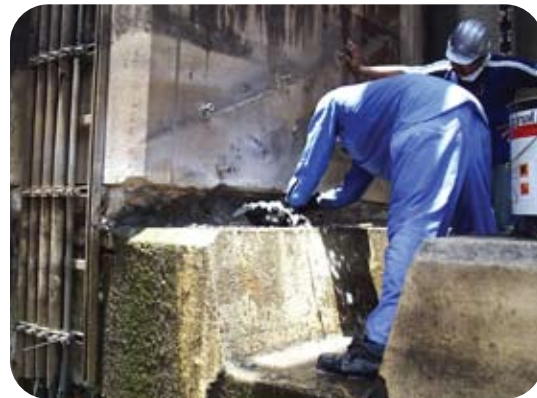
Severe leakage of Dubai drydocks before Krystol Crack Repair System was applied
