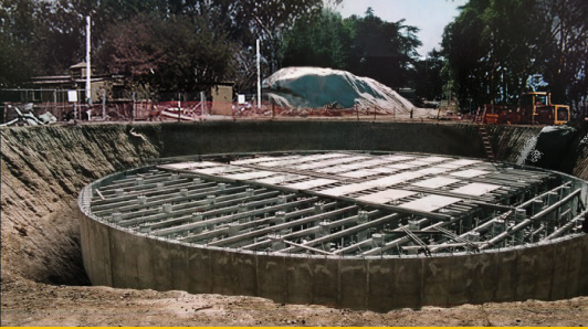
TreePeople Center Rainwater Cistern, Los Angeles, USA
